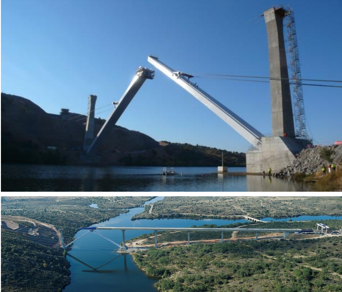
Fig. 12. View of the tilting manoeuvre and the deck launching over the arch
