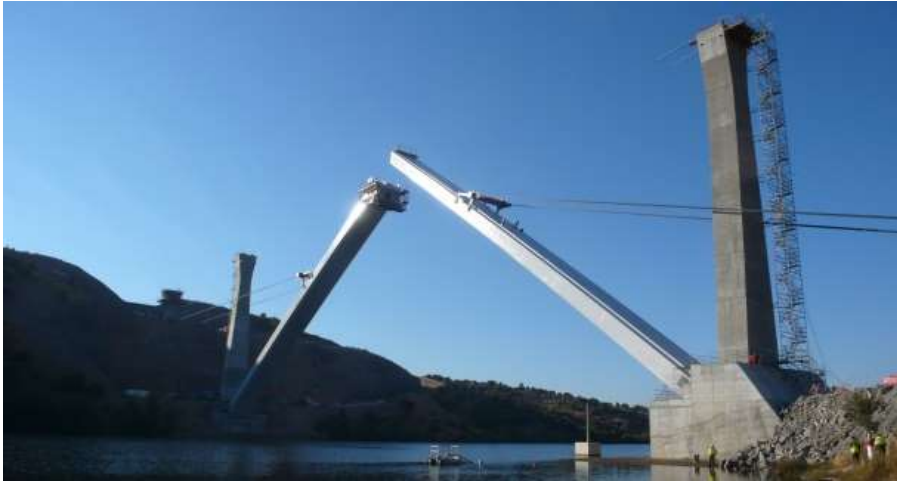
Fig. 12. View of the tilting manoeuvre and the deck launching over the arch
